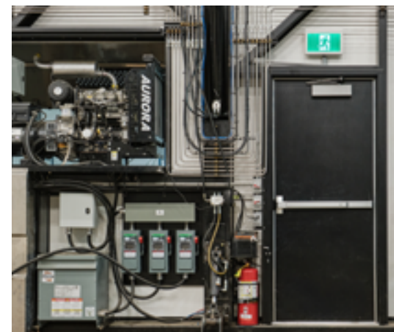
600V 3-phase AURORA generator
